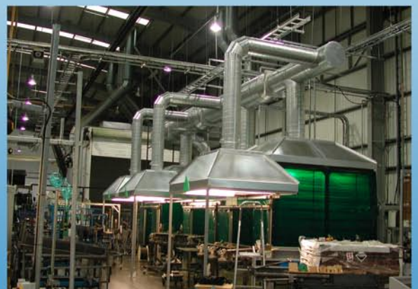
Fume Extraction System
